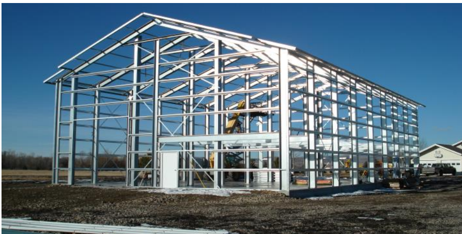
A cold formed steel building project erected by TNT Construction in Montana.
